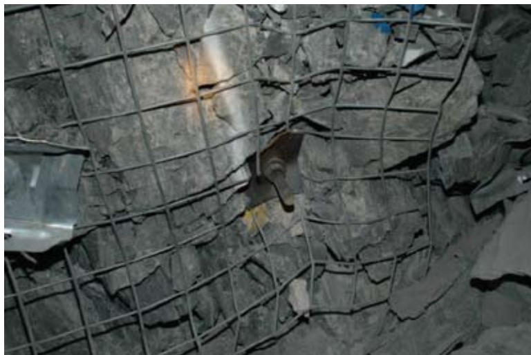
Support damage after blast testing performed in Phase 3
