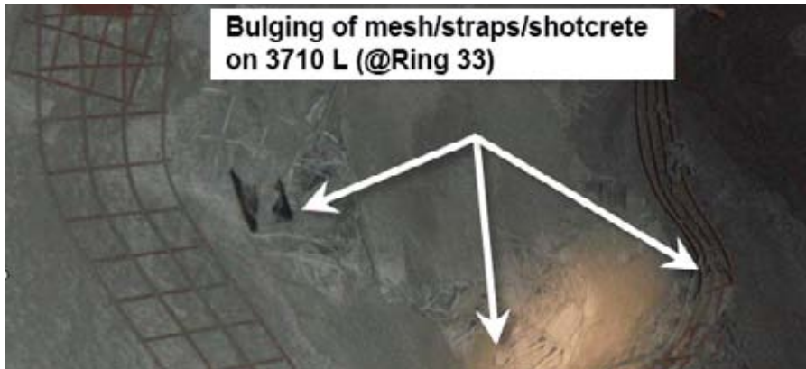
Figure 5 Minor cracking and bulging of the support system following a 2.3 Mn event in 9280 top sill
