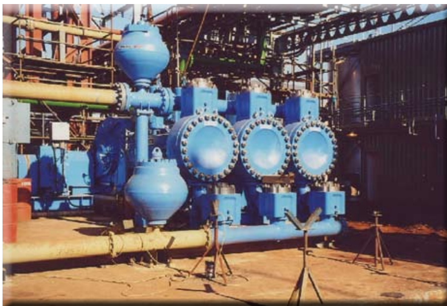
Positive displacement pumps at Richards Bay (Hillendale)
