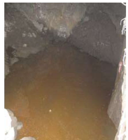
Figure 25 Water draining through the barricade, SNM stope
